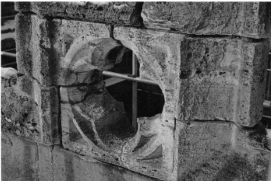
Figure 2.6 Mortar eroded out of medieval masonry through wind action.
