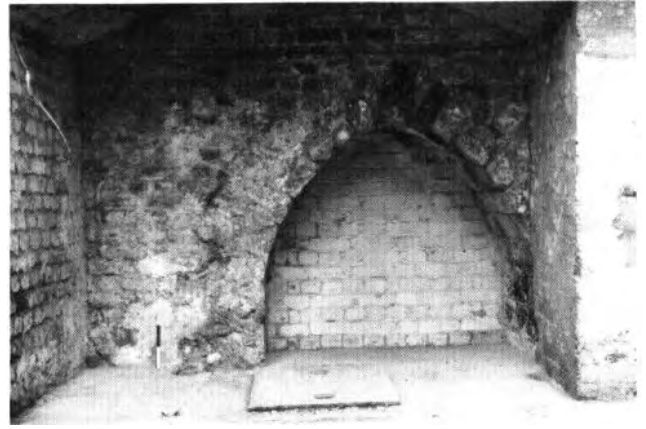
Fig 116 15-35 Copthall Avenue, watching brief: blocked-in medieval culvert on London Wall frontage. Scale in 0.10m units
