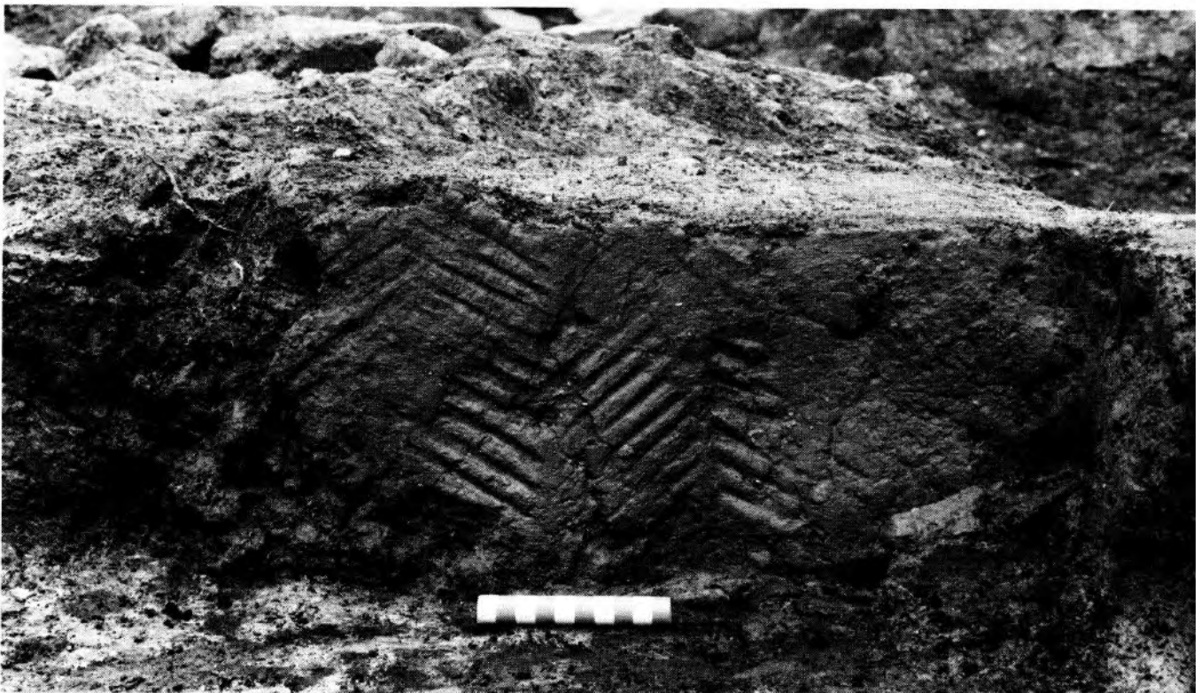
Fig 71 Newgate Street: detail of the chevron pattern impressed into the south face of the wall between rooms iv and v in Building K (Period VII.9; Fig 13). Scale in 10mm units.
